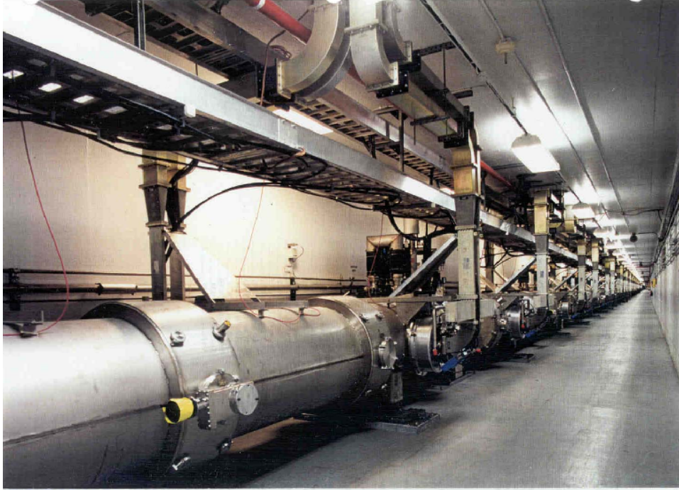
Figure 2.5: Linac's assembly with its cryomodules inside the beam tunnel. Image source [32].
